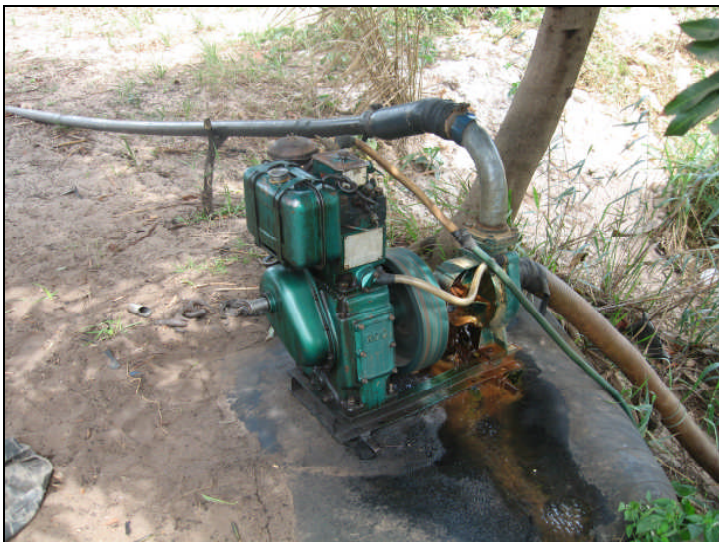
Plate 3.7 Typical water pump.
